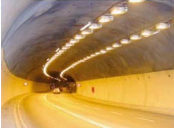
Fig. 6: Application of white cement-based panels reduces need for lighting in underground tunnel.
