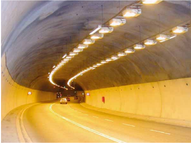
Fig. 6: Application of white cement-based panels reduces need for lighting in underground tunnel.
