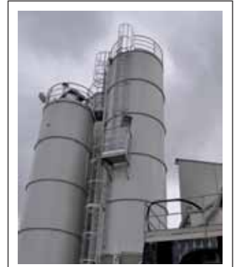
Ready-mixed concrete plants
